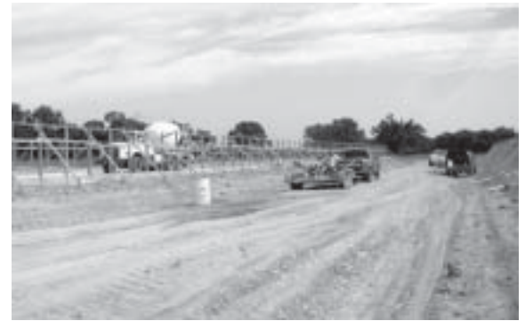
UNDERWAY - Construction has started on the new facility Cobb-Vantress is financing for the U of A.
